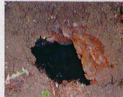
An inspector found this barrel was being used as the septic tank and even the metal lid was corroded.
